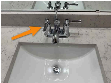
Primary Bathroom Right hot water
