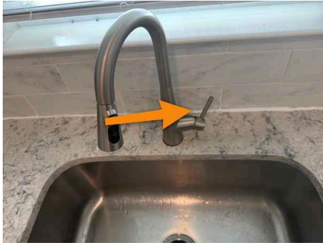
Kitchen hot water
