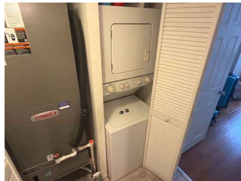
Laundry Closet- Operated
