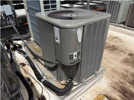
Refrigerant line intact
